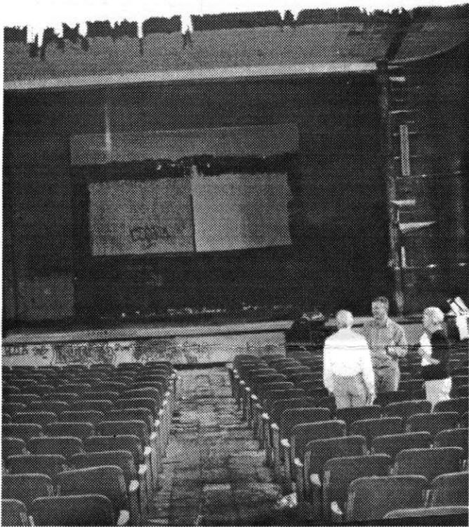
The Auditorium of the Junior High School slowly deteriorates from neglect and vandalism. Photo by Richard McClelland.
